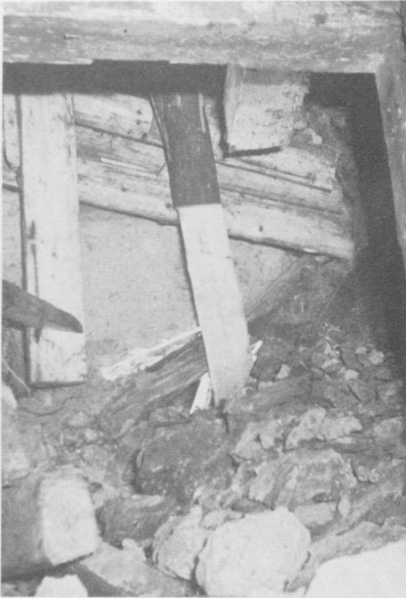
Fig. 54 Rockburst of January 29, 1943; 3801W Drift looking west from Sec. 6.5W.
