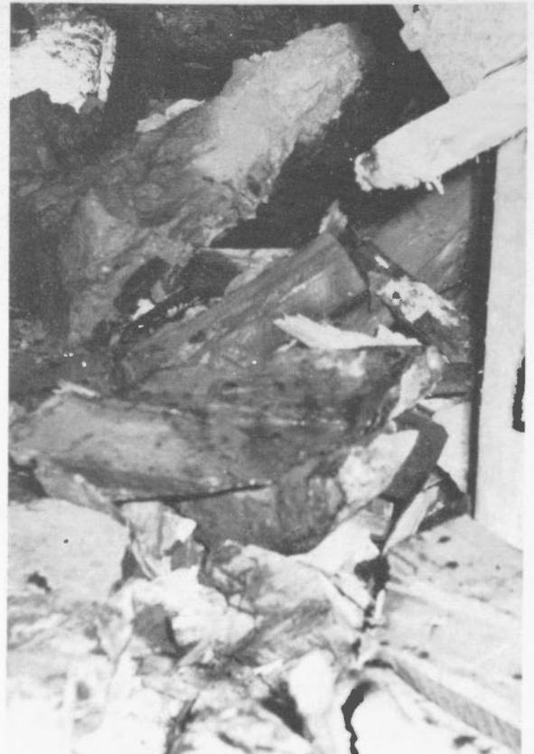
Fig. 55 Rockburst of January 29, 1943; 3901W Drift, looking west from Sec. 6.5W.
