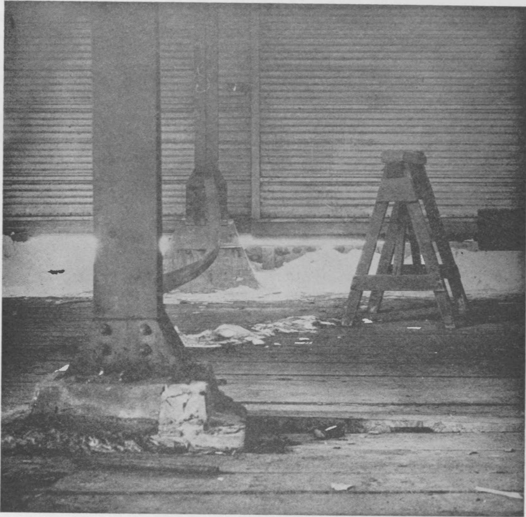
FIG. 9.—Bent back brace at freight sheds at Quebec
