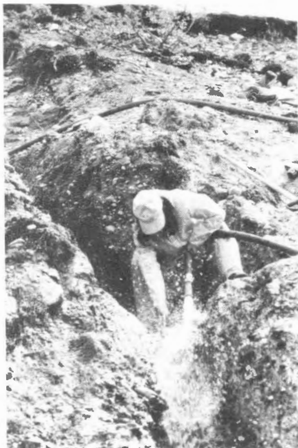
Using portable high-discharge fire-fighting pump to create clean stratigraphic exposures of perennially frozen till, Kazan River, District of Keewatin.
