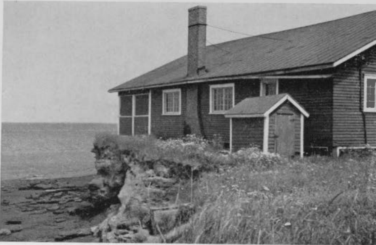
Figure 11. The cottage is threatened by the sea as the erosion face has retreated to within inches of the structure.
