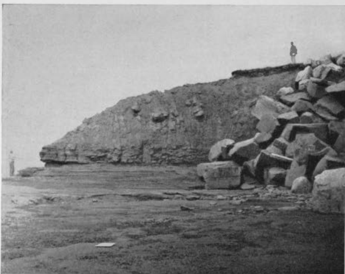
Figure 6. This narrow headland is suffering severe wave attack. The rock has been undercut and the bouldery till has been removed in large quantities, leaving the surface sod well back from the rock face. The large, quarried sandstone and granite blocks on the right have been placed there to check erosion.
