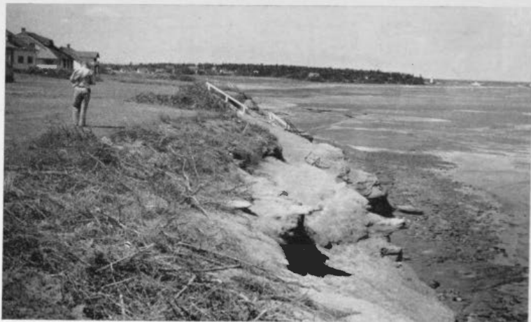
Figure 12. The placement of tree branches along the erosion face of unconsolidated material overlying rock is an attempt to retain the soil.
