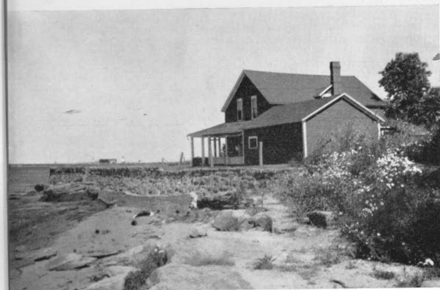
Figure 15. This stone and concrete retaining wall protecting a house is well maintained and quite durable.
