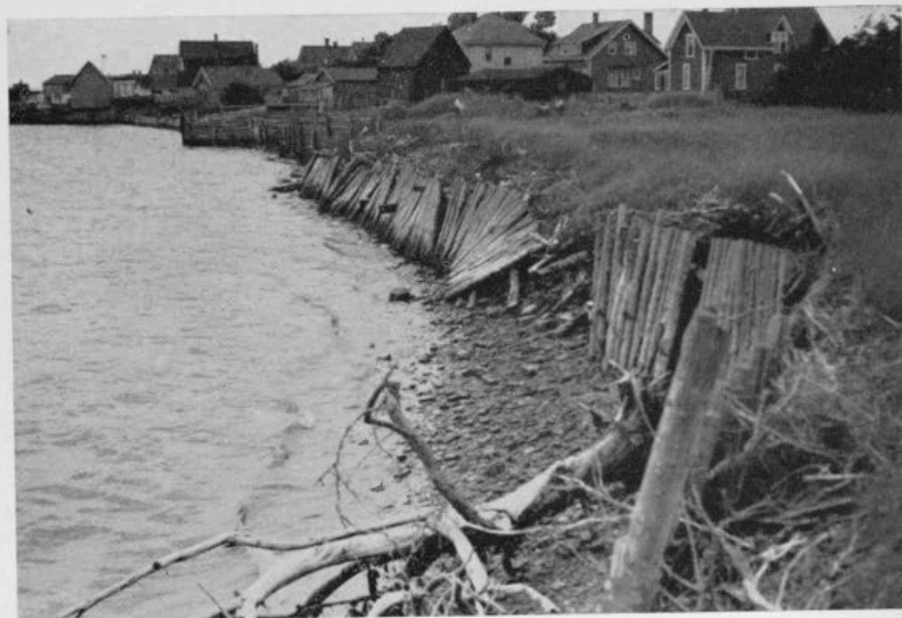
Figure 14. This wall of vertical posts has been so badly damaged that it is completely ineffective.
