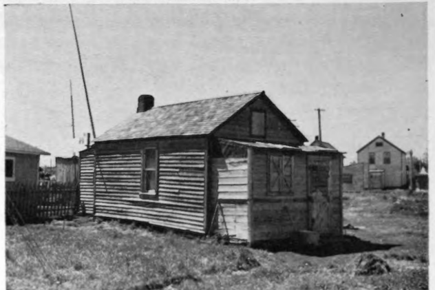
Figure 12. A class D house. Homes of this type are little more than shacks. They are generally small, unpainted frame structures, badly built and poorly maintained.
