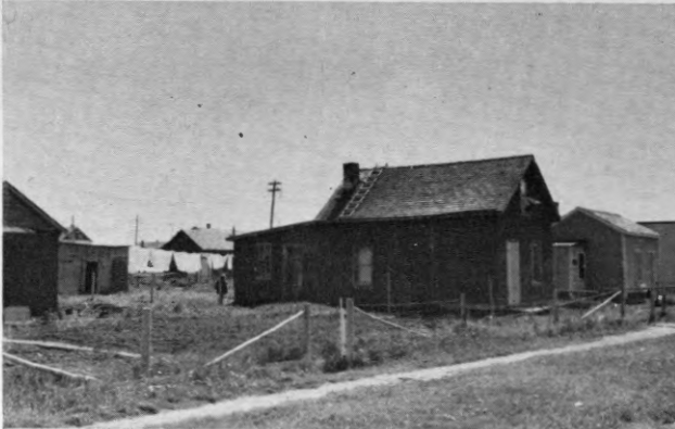
Figure 11. A class C house. A poorly constructed frame building covered with brick siding.
