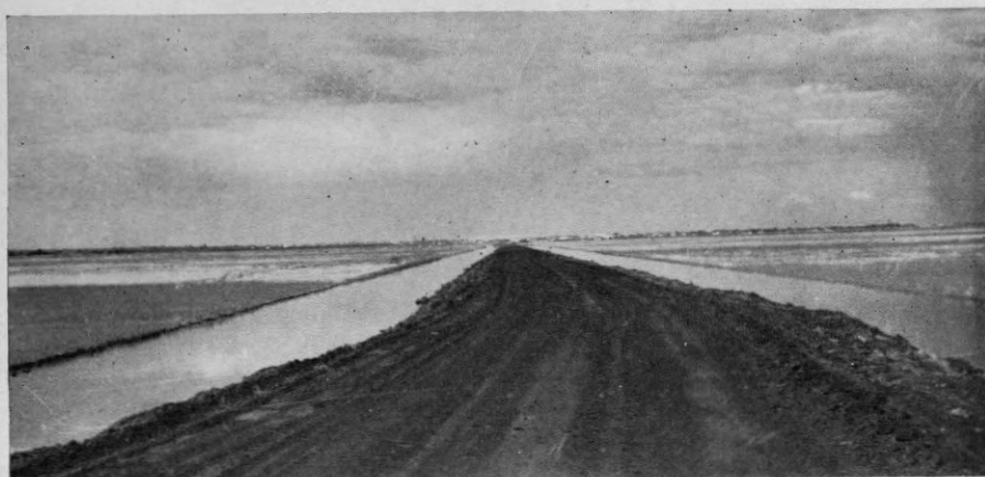
Figure 5. A newly built road in the lowland of the Pasquia and Carrot Rivers. Note the low relief, absence of trees or shrubs, and abundance of water.
