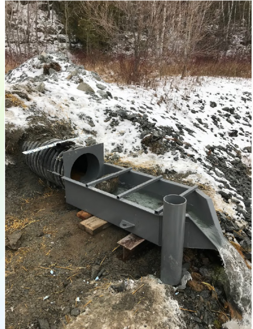
H-Flume at Shaft #98
