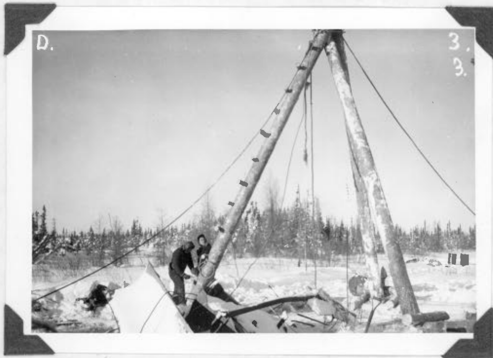
Another view of tripod over sunken bulldozer
