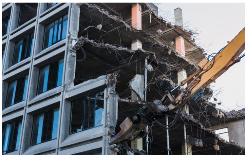
Figure 2: Demolishing of a building destroyed by the earthquake of 2011 in Christchurch, New Zealand (Photo: KiraVolkov/istock).
