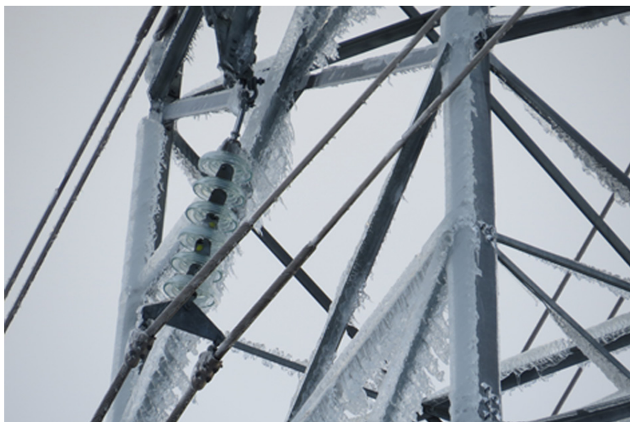
Figure 1: Ice buildup on electrical infrastructure (Photo: BC Hydro).
