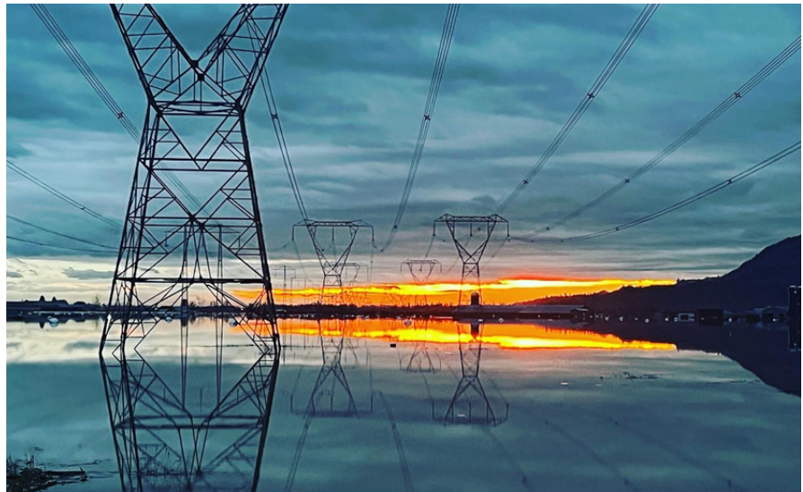
Figure 3: Electrical infrastructure in the Sumas Prairie during November 2021 flood (Photo: Lizz Koebel-Davidson).
