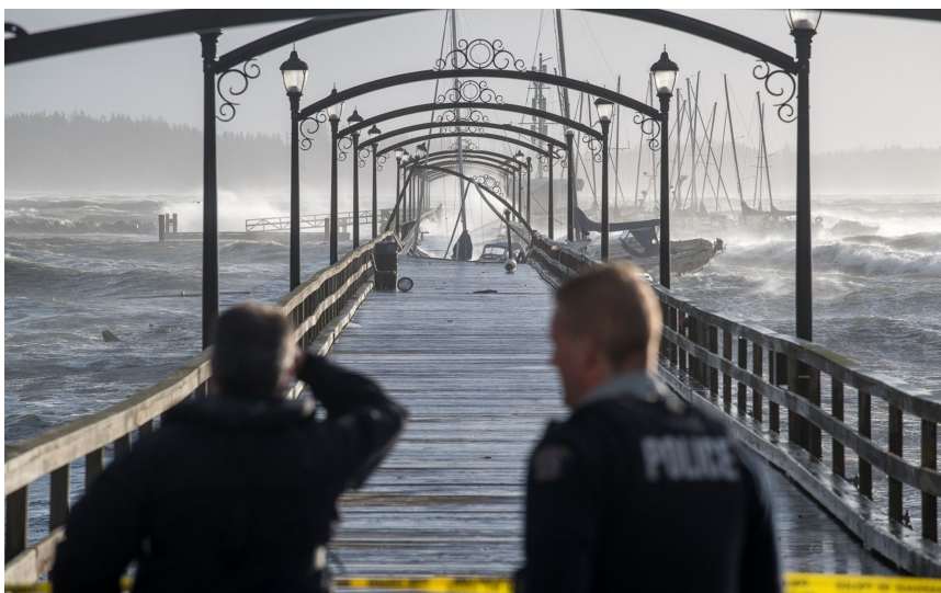
Figure 2: White Rock Pier Collapse, December 20, 2018 (Photo: Tim Shields).
