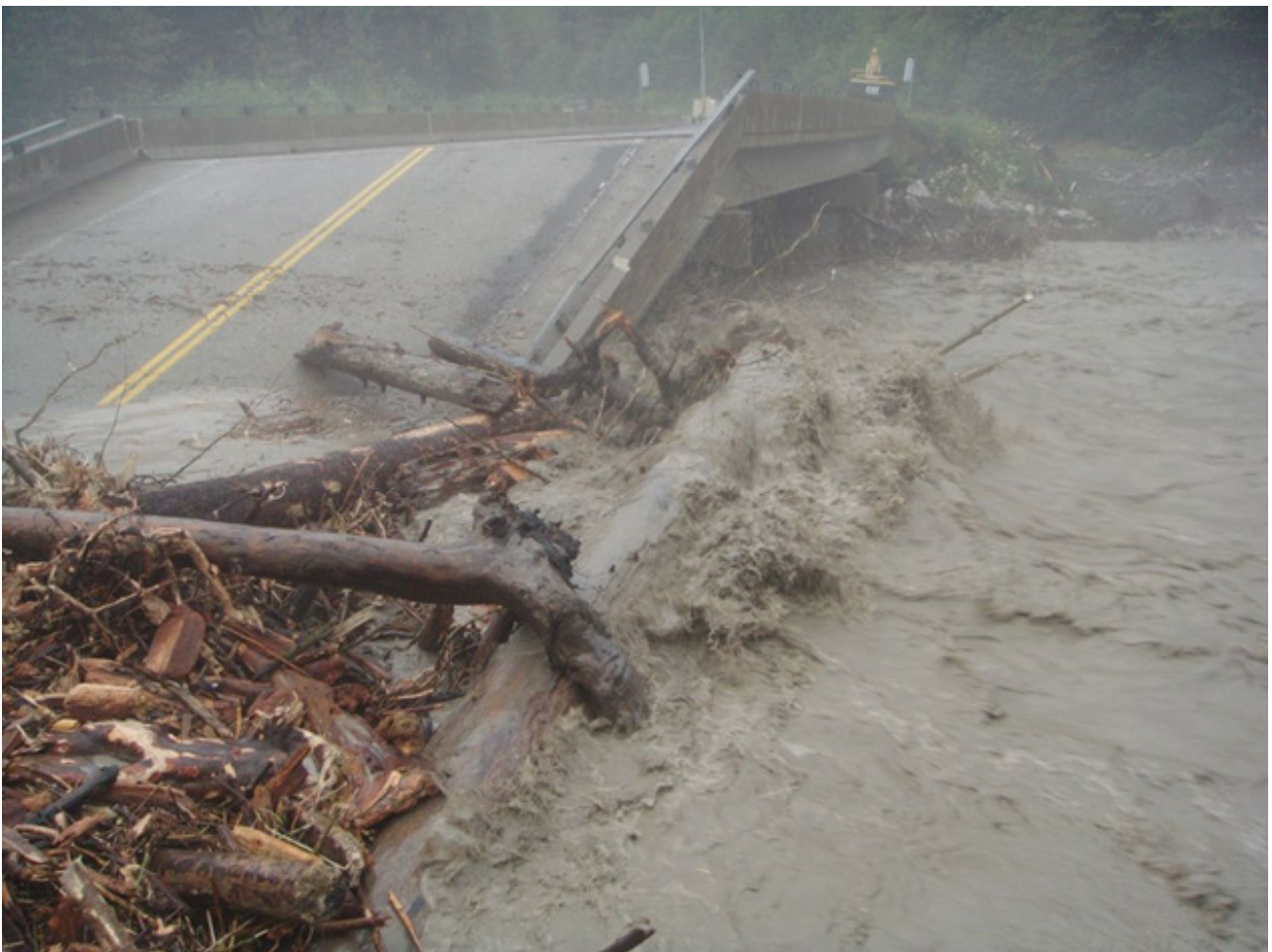
Figure 10: Stewart: Highway 37A Flood Impacts – Bitter Creek bridge failure. (Source: British Columbia Ministry of Transportation and Infrastructure)
