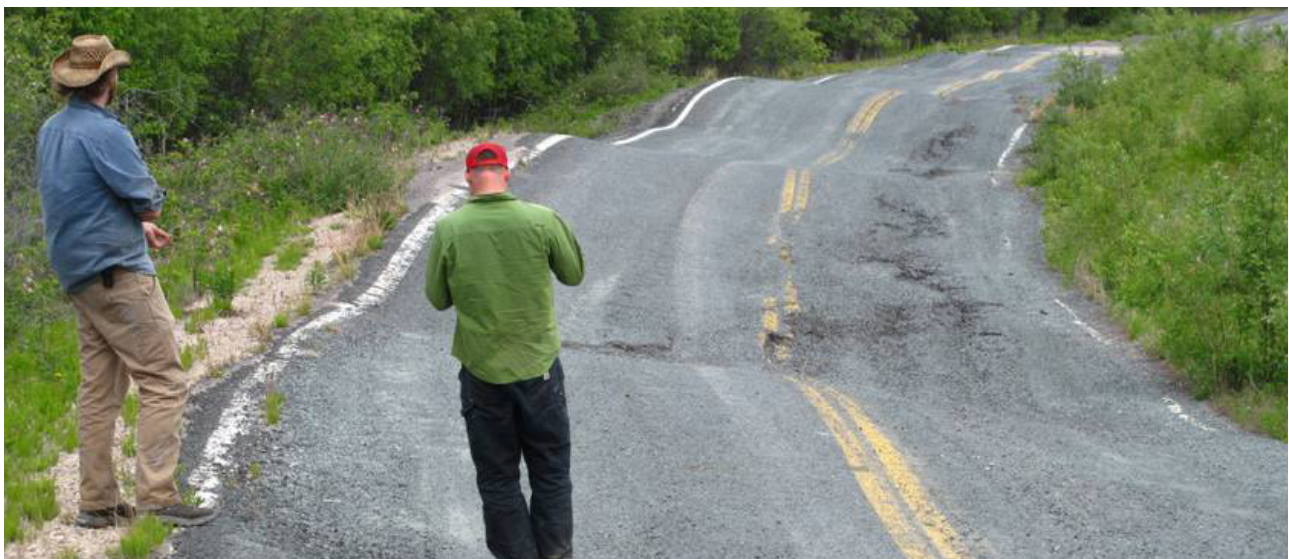
Figure 7: Differential settlement associated with permafrost thaw along an abandoned section of Northwest Territories Highway 4, east of Yellowknife. (Source: Natural Resources Canada)
