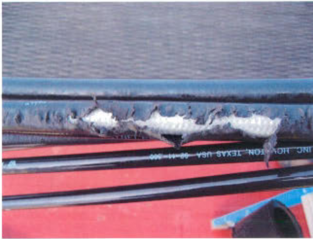
Damaged air hose.
