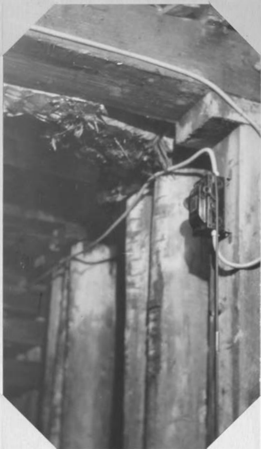
Fig. 12. Wiring to Set-up on the 2950-foot Level
