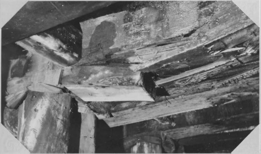
Fig. 10. Beam Crushed by End Thrust in 2950-foot Level
