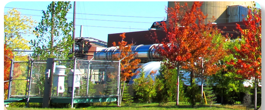
Stop 1: Air quality monitoring station in the Little Italy park beside the Copper Cliff smelter.
