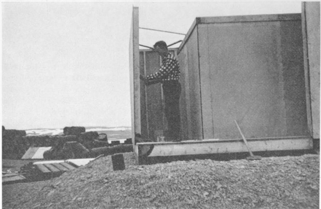
FIGURE 7—The recorder building under construction. The inside recording room has been completed and the outer protecting building is being erected.
