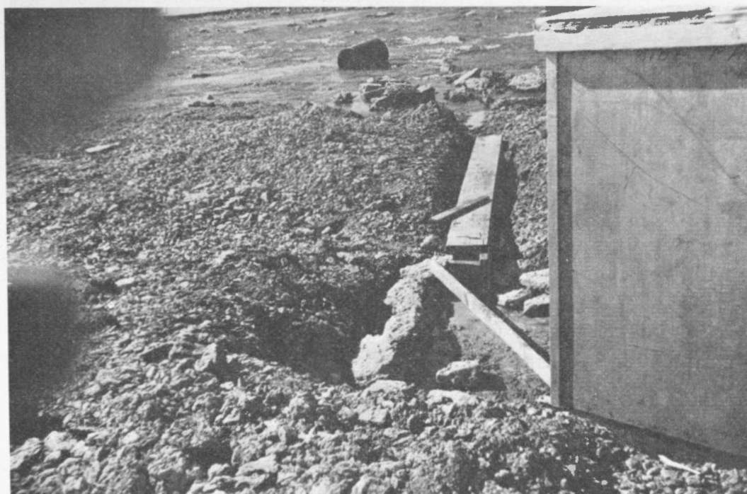
FIGURE 2—Drain for carrying away the water from the disturbed permafrost. The large stones prevent gravel from blocking the passage of water.
