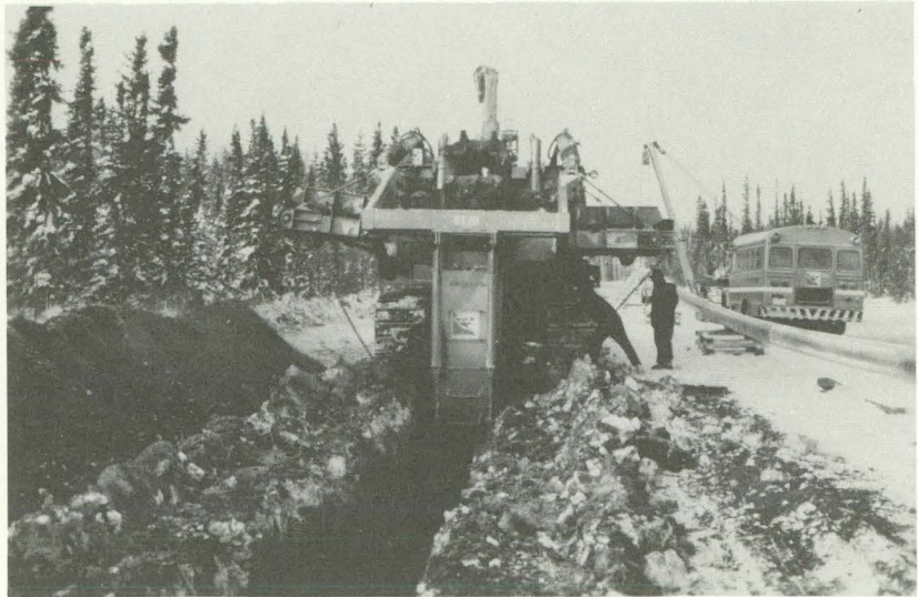
Arctic ditcher, excavating trench through organic terrain north of Fort Simpson (January 1984).
