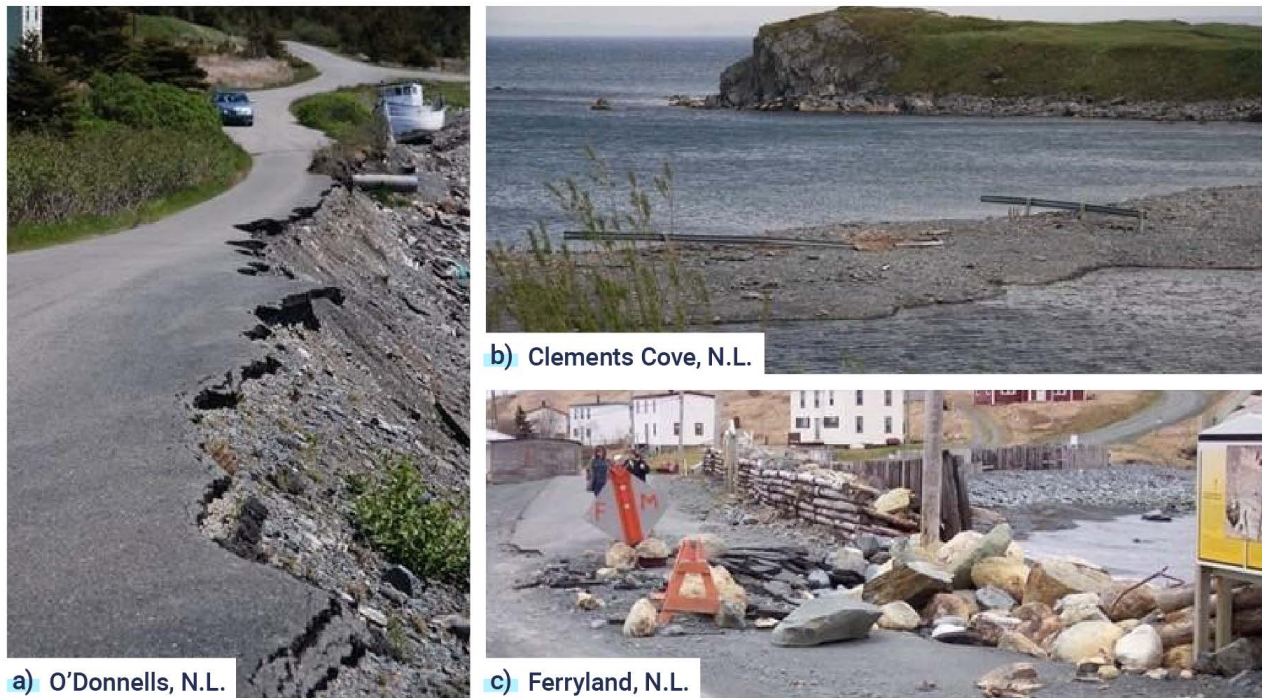
Figure 1.7: Three examples of vulnerable coastal roads in Newfoundland and Labrador. a) Dead-end road that extends west from the community of O'Donnells, Newfoundland and Labrador, which was eroded following several storm events between 2007 and 2011. The road is no longer being maintained. b) The road that formerly followed the crest of the barachois in Clements Cove, Newfoundland and Labrador, which has now been abandoned following several wash-over events that took place between 1990 and 2010. The displaced guardrails remain. c) The breakwater that protects the tombolo road in Ferryland, Newfoundland and Labrador, was damaged frequently as a result of storm events between 1989 and 2010, and necessitated periodic reconstruction and maintenance. Photos courtesy of Norm Catto, Memorial University of Newfoundland.
