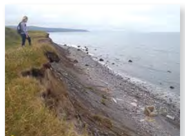
Point Verde, 2011. Structure now on beach.
