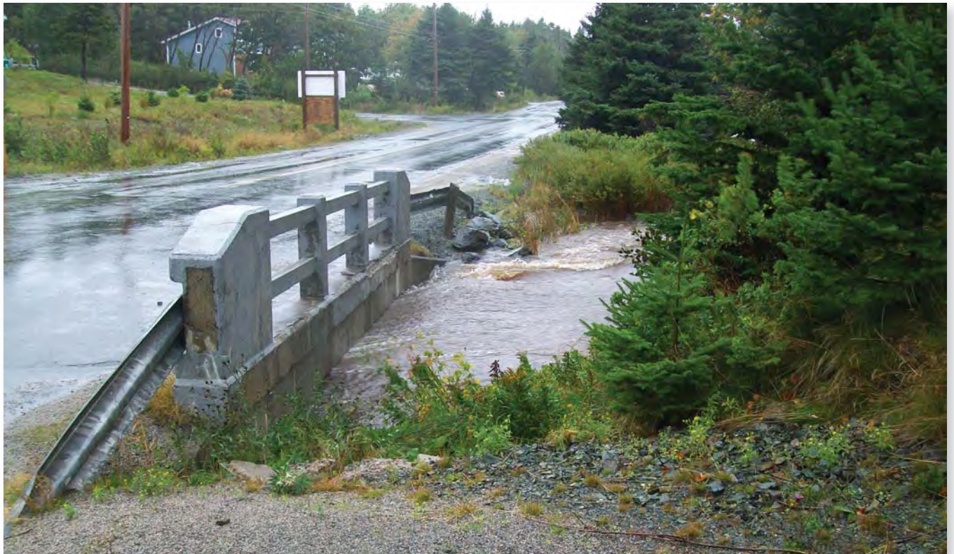
Figure 3: The Savage Creek Bridge over Outer Cove Brook floods regularly, as seen here following Hurricane Igor. The bridge is slated for replacement.
