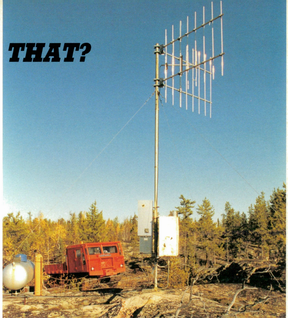
Array outstation showing transmitting antennae and electronic boxes on mast. Tank on left supplies propane for thermoelectric generator
