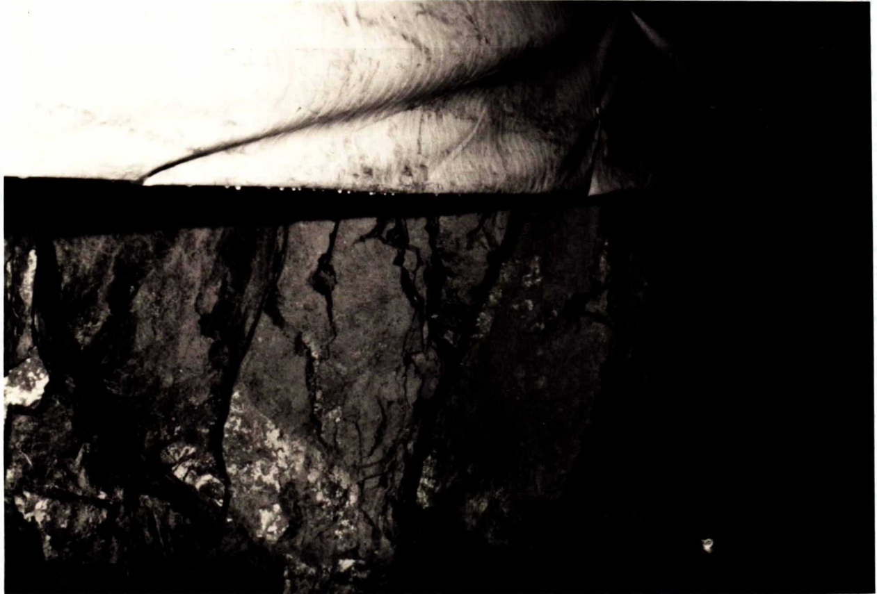
Figure 12 Potential toppling prism failures.
