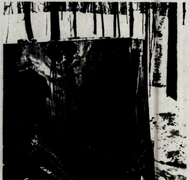
Figure 11 - Heat caused door to warp
