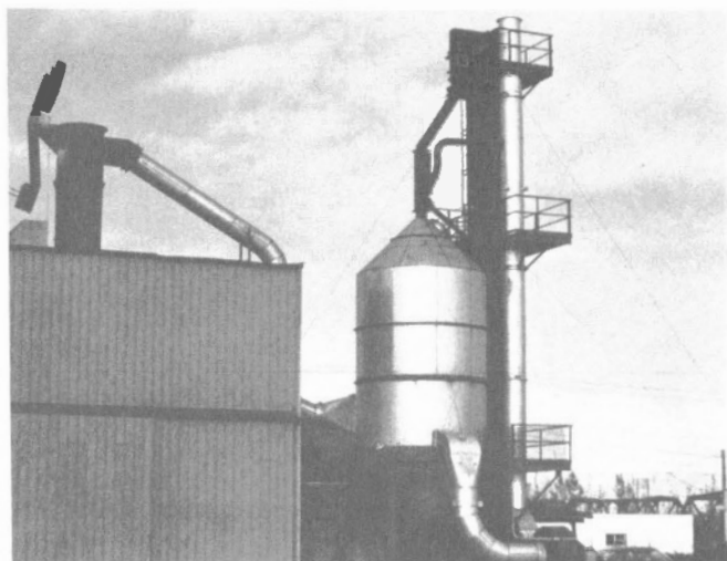
Packed-bed filter and stack at Thor Foundry Ltd., Winnipeg
