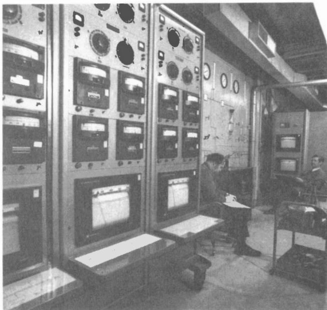
M.P. Pleet and R.W. Beer of Fuels Research Centre supervise continuous run of hydrocracking plant
