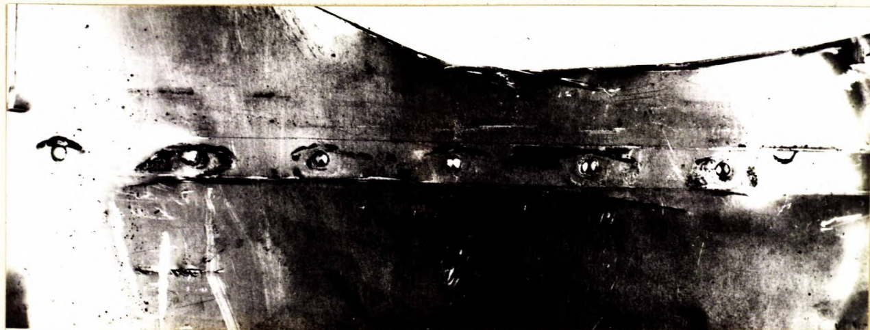
INSIDE VIEW OF THE CRACKS. (Approximately 2/3 actual size).
