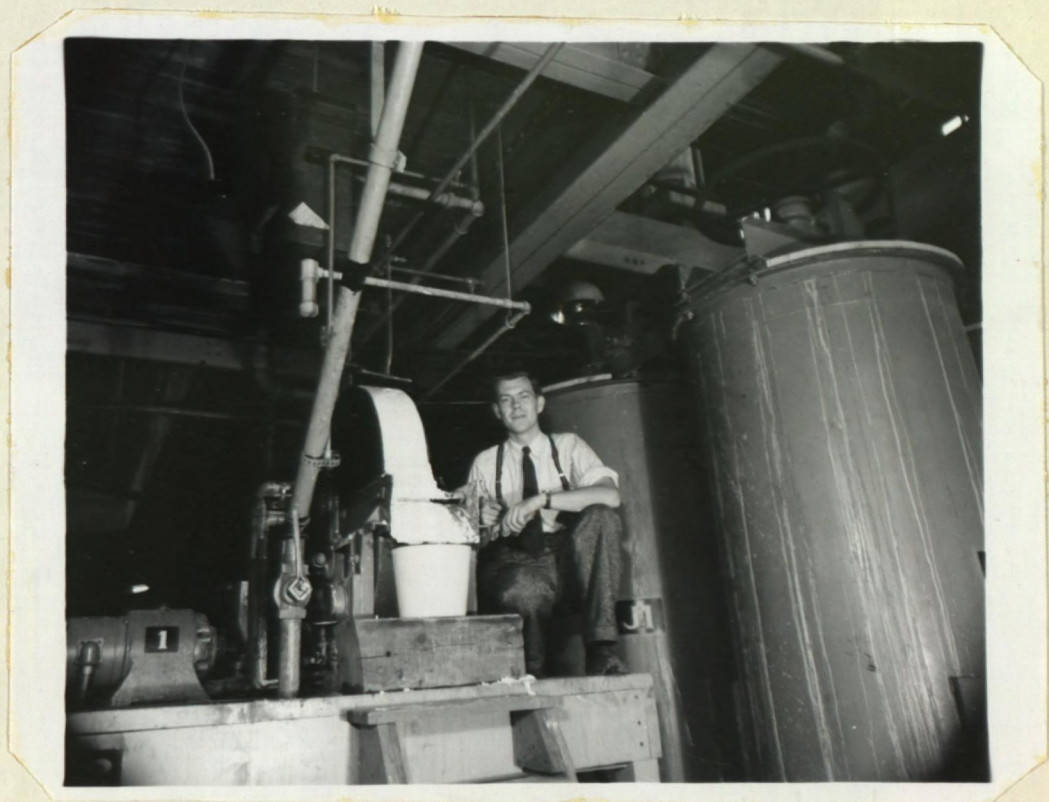
Oliver filter, showing discharge of alumina hydrate product. Alumina precipitation tanks shown on right.
