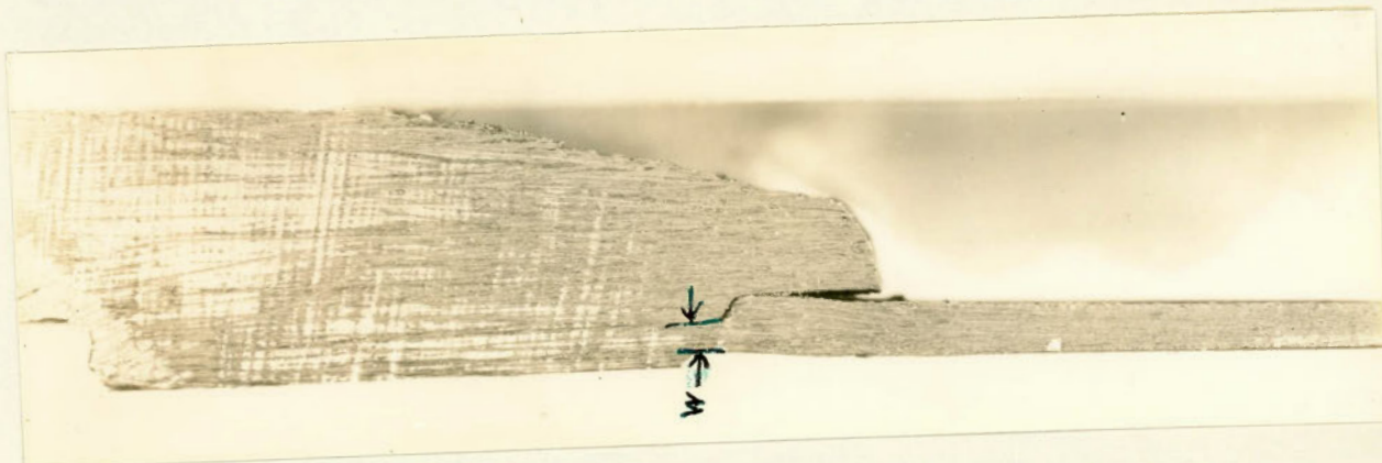
A close-up of the welded joint, showing the extent of the weld, dimension "W".
