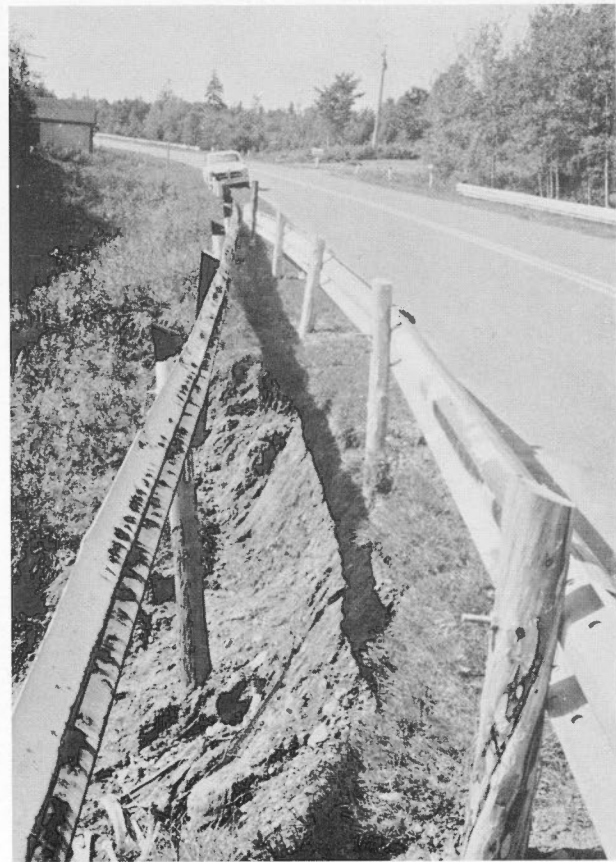
FIGURE 17. East Point Road, Route 16, eastern P.E.I. An example of very severe erosion on a steep roadside slope. Note the old guard rail on the left and the new rail on the right, demonstrating the extent to which the embankment has been eroded. Note also that the new guard rail is beginning to be affected.
