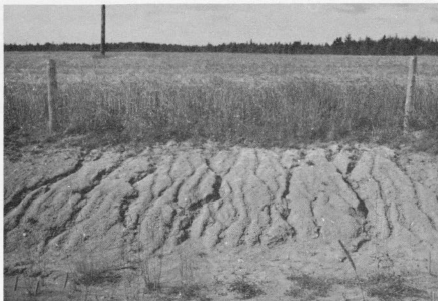
FIGURE 4. Western Road, western Prince County, near Carleton. Rill erosion (Class 2) on the backslope.
