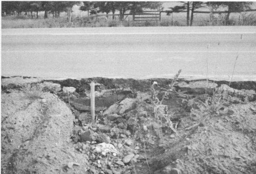
FIGURE 23. Trans-Canada Highway, near Vernon, eastern P.E.I. Notable deterioration of the paved highway shoulder and the roadside area. This gully is 11" deep and 3' wide.
