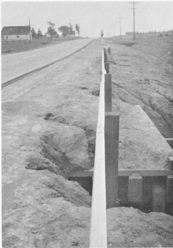
FIGURE 16. Western Road, western Prince County, near Richmond. Advanced erosion (Class 5) encountered at bridge structure. Note the extension of gullies inside the guard rail. One gully measures 3'6" in depth and 5' in width.
