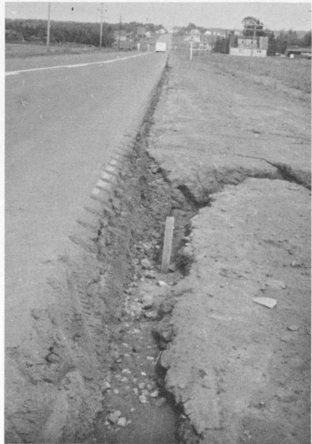
FIGURE 22. Western Road, western Prince County, near Richmond. The development of unsafe motoring conditions due to gully-ing parallel to the edge of the pavement.
