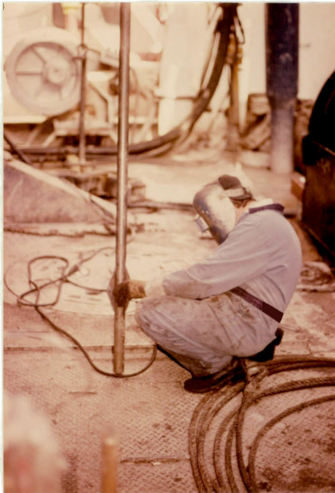
11. Welding on centralizer fins on the bottom of the sinker bar. Panarctic welder. (C16)
