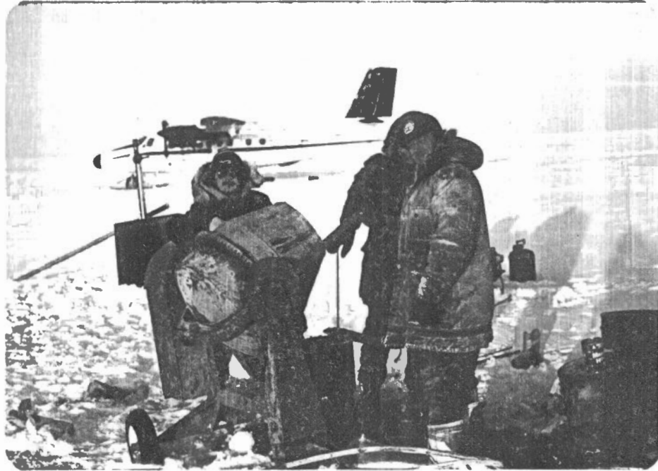
Placing cement surface plug at final abandonment by Earth Physics Branch, EMR, May 1, 1982.
