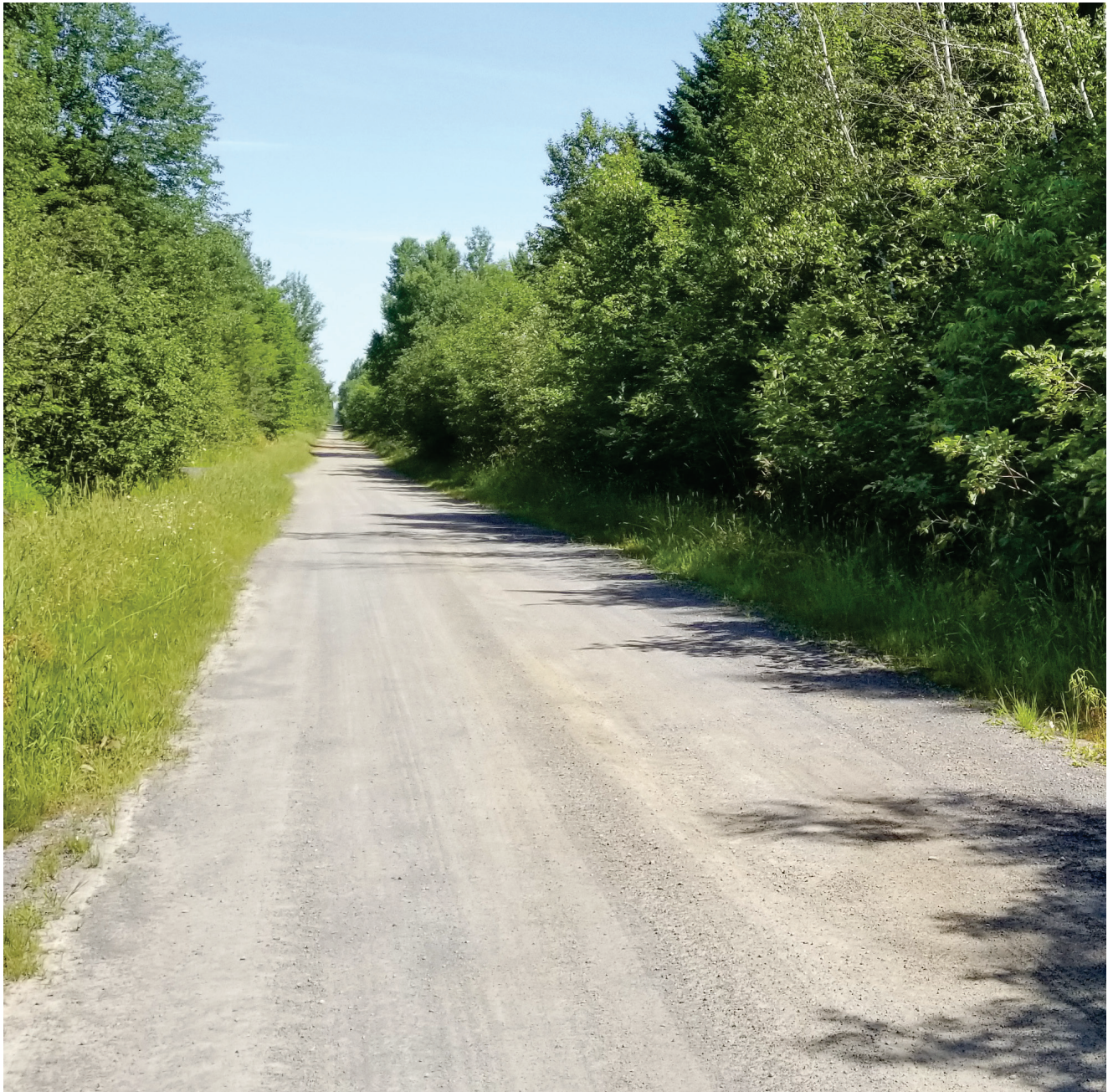
Fig. 3 Photo of Canaan Road at Cheney landslide site (Taken July 4, 2018 at CT15, facing north. See Fig. 2 for location.)
