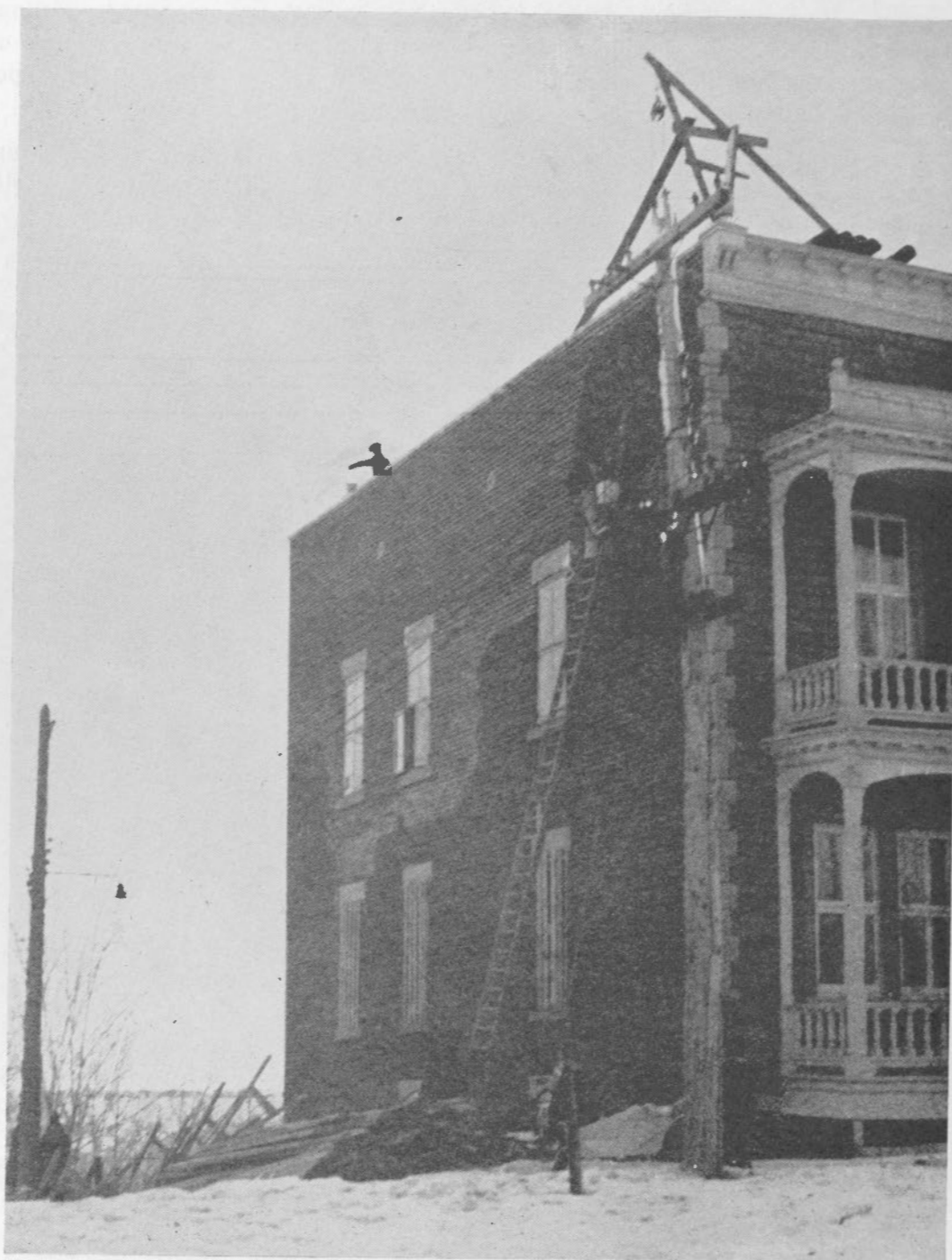
FIG. 13.—Damaged wall at Shawinigan Falls
