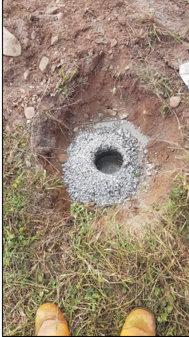
Figure B.3 - PO-01 during at the final stage (step 5) of the decommissioning (August 24, 2018)
