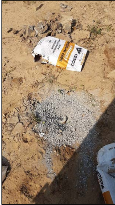
Figure B.21 - Observation well PO-08 in the decommissioning final stage (step 5) (August 25, 2018)
