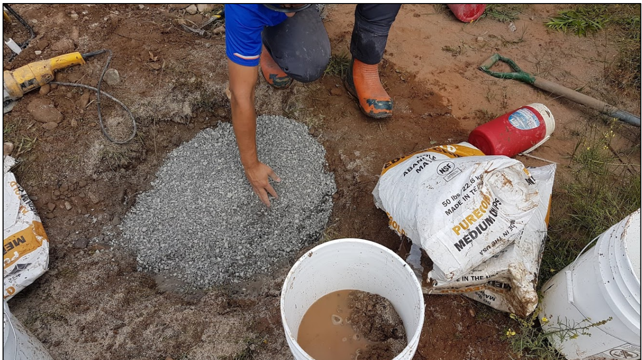
Figure B.28 - Observation well PO-13 in the final stage (step 5) of its decommissioning (August 26, 2018)
