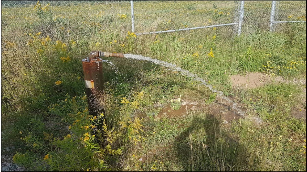
Figure B.5 - Observation well PO-02 showing artesian condition before its decommissioning (August 26, 2018)
