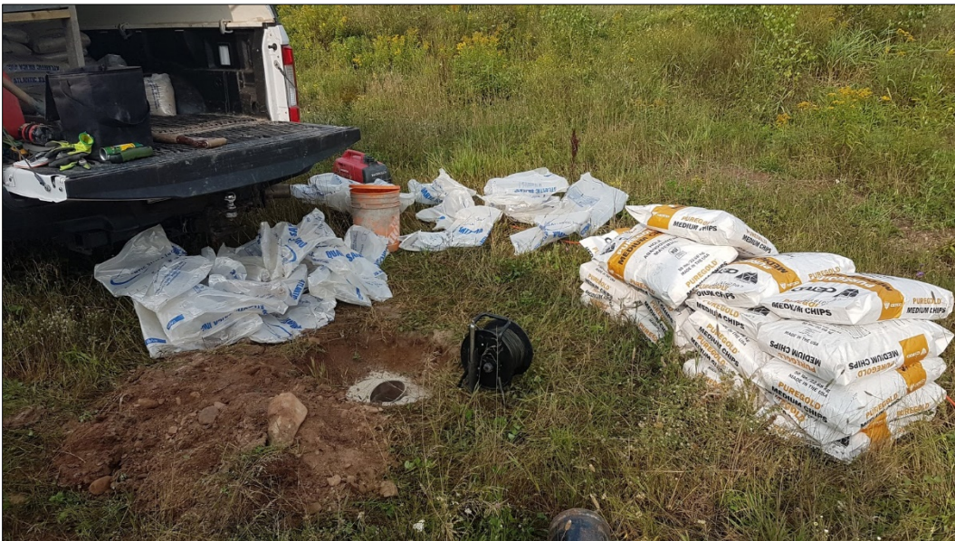
Figure B.2 - Observation well PO-01 after the casing was cut at 60 cm below the ground surface (step 2) (August 24, 2018)
