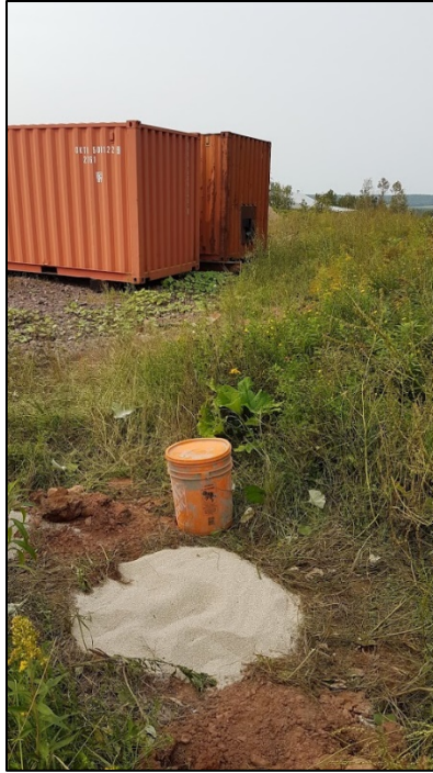
Figure B.17 - Observation well PO-07 at the final stage of its decommissioning (August 24, 2018)
