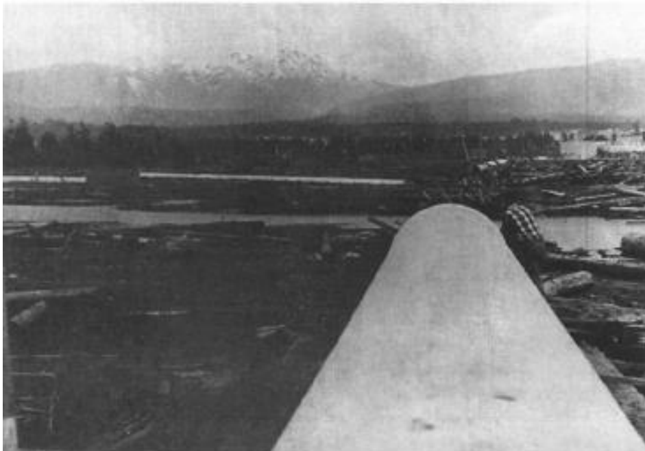
Figure S3-3 Breached water pipeline on the Somass River delta shortly after the 1964 tsunami. Source image: Port Alberni Museum photo 4383 (from Clague and Bobrowsky 1994).
