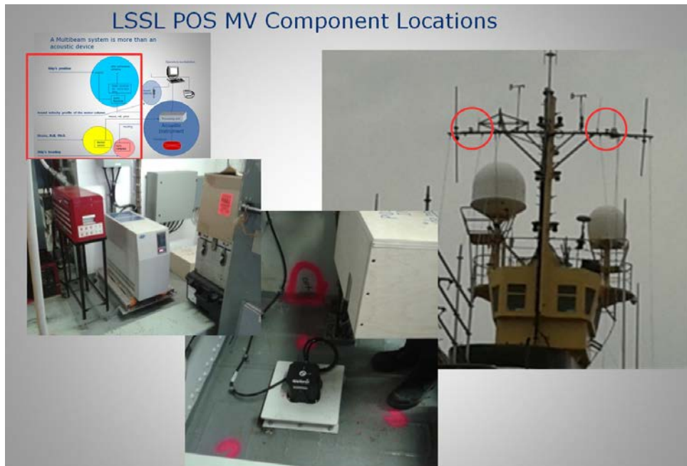
Figure 2.6. Locations of various components of the EM system. The two POS MV antennae are located on the ship's mast and the Inertial Motion Unit (IMU) is located in the Emergency Generator Room,
