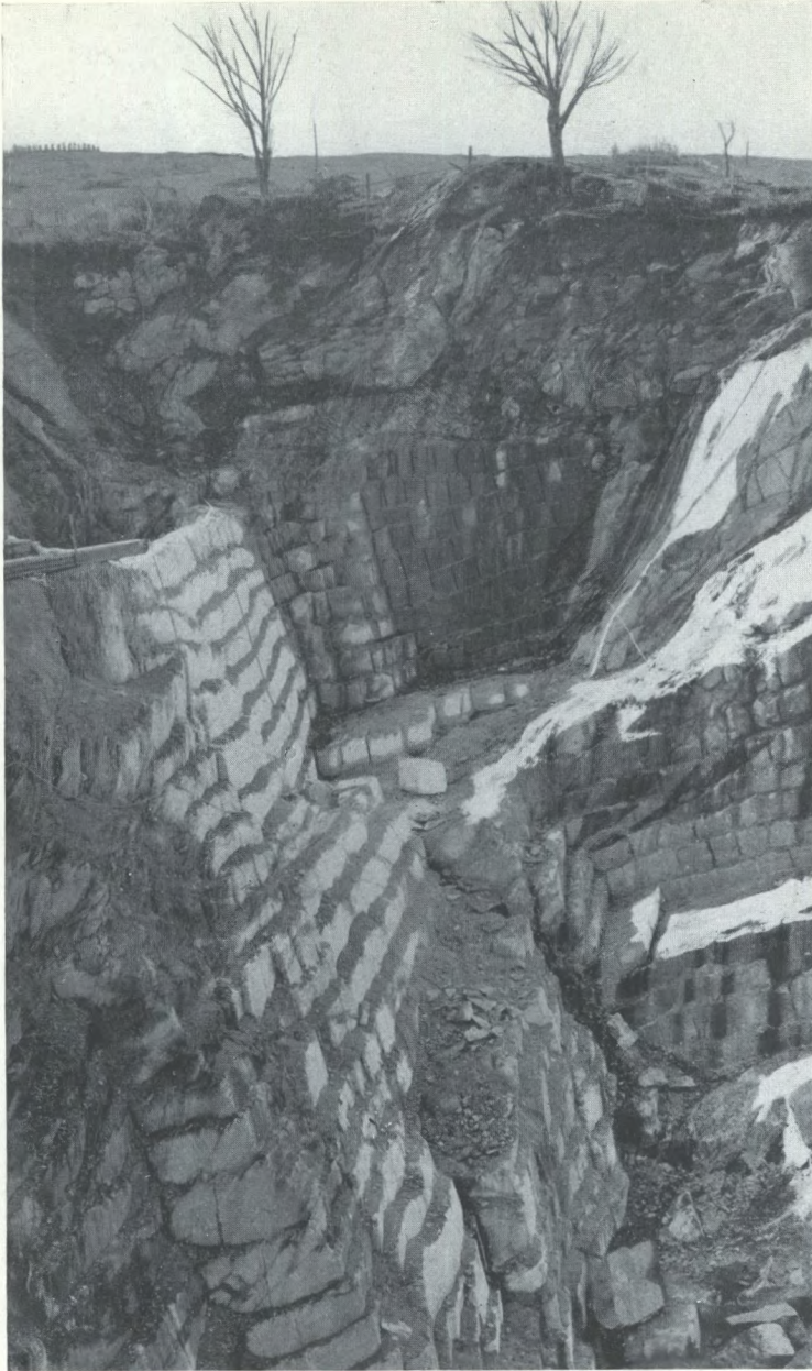
View of soapstone quarry of Broughton Soapstone and Quarry Company, range XI, lot 12, Broughton Township, Beauce County, Que., showing method of drilling out the stone in blocks along rough benches. The opening measures 250 by 225 feet and is 75 feet deep.
