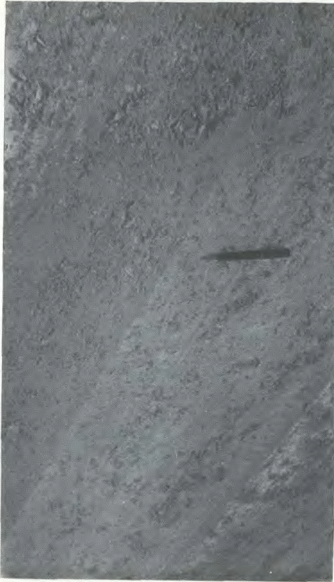
A. Close-up view of stabilized road surface: sodium chloride treated road at Cookstown, Ont.
