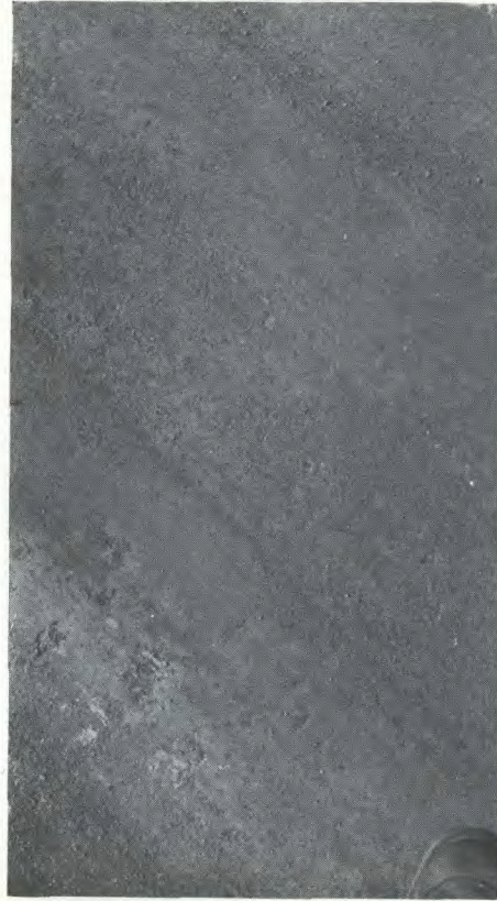
B. Close-up view of stabilized road surface: calcium chloride treated road between Huntsville and Dwight, Ont.
