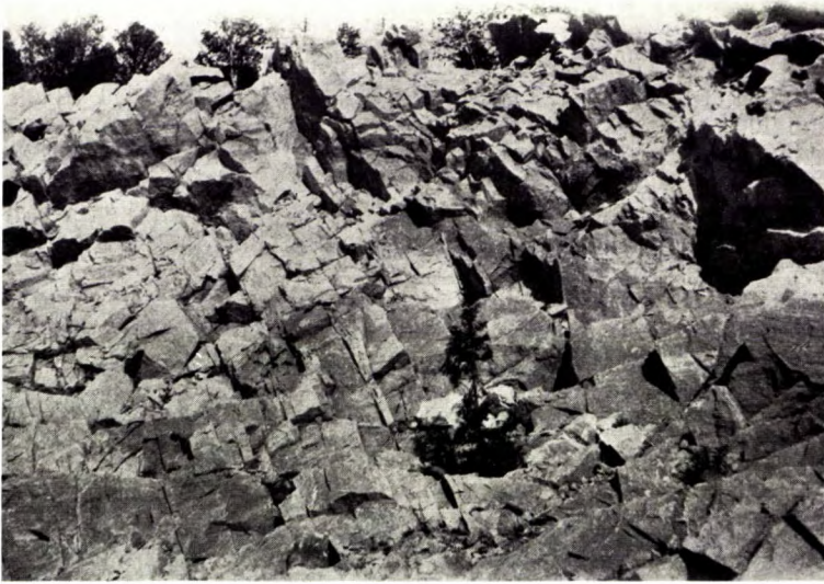
A. Drury Cove quarry, Drury Cove, St. John County, N.B., showing the irregular jointing characteristic of most of the Precambrian limestones of the district.
