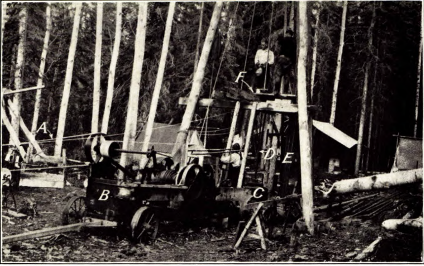
A. Equipment for core-drilling Alberta bituminous sand: A, belt to tractor; B, portable well drilling rig; C, rotary table; D, drill rod; E, drill rods not in use; F, platform for connecting and disconnecting drill rods.
