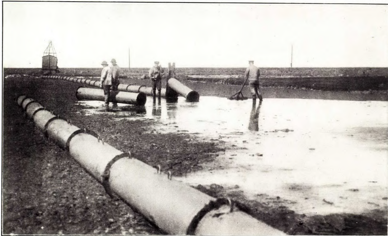
View on drying-ground showing movable pipe sections used for spreading raw peat in the hydro-peat process
