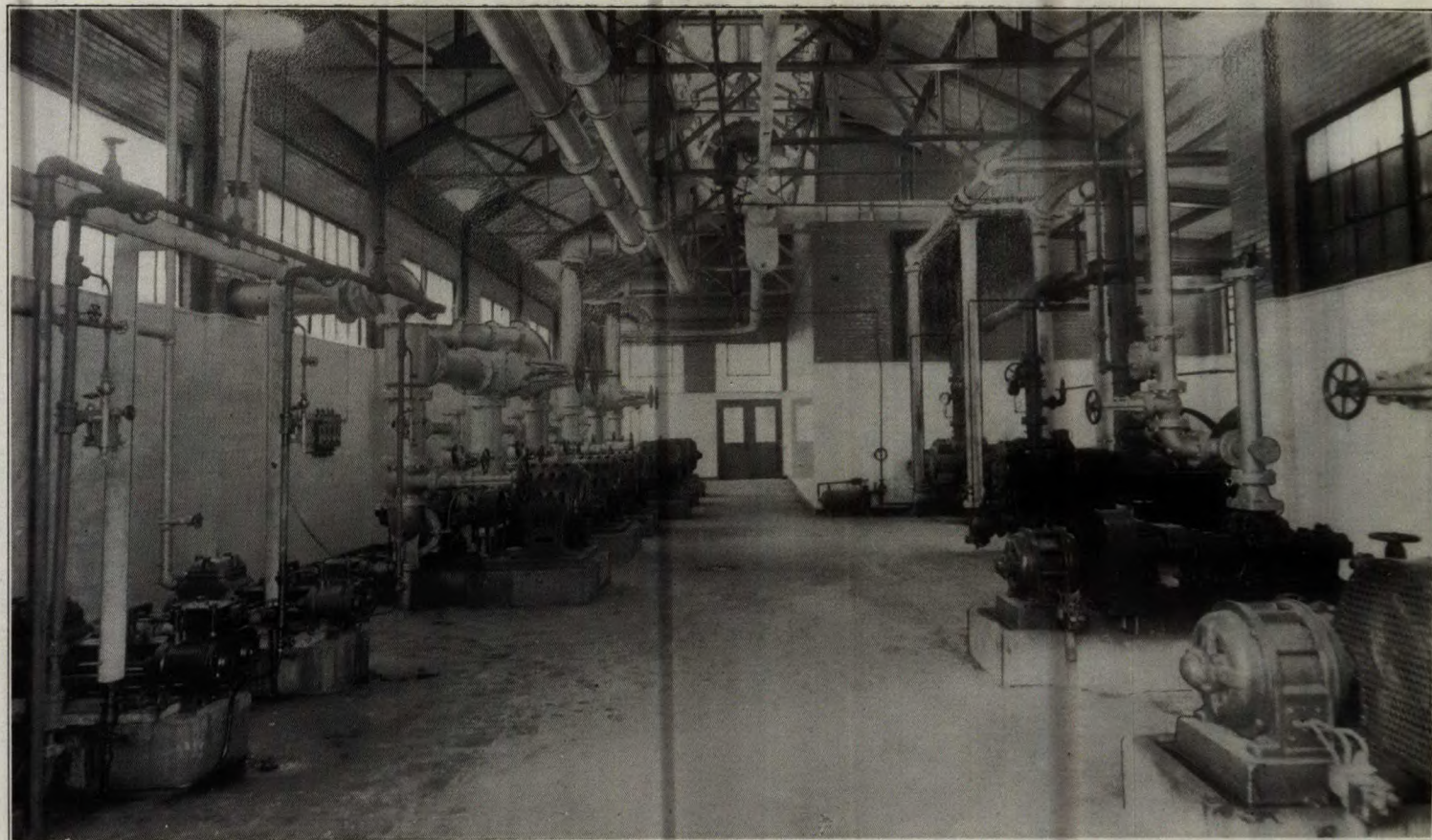
Typical pump-house installation.
