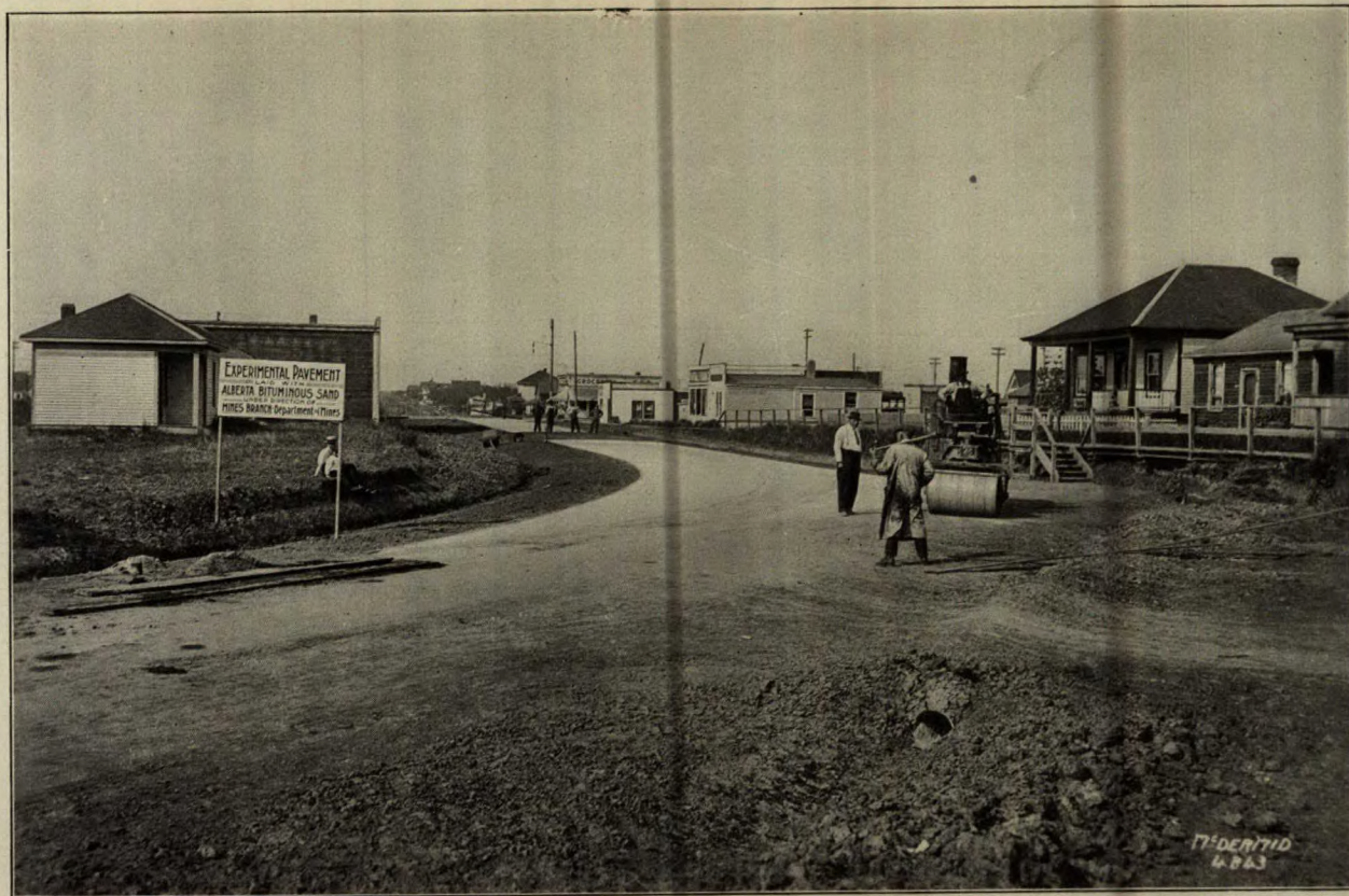
Bituminous sand pavement laid in Edmonton, Alberta., under supervision of S. C. Ells, Mines Branch, August, 1915.
