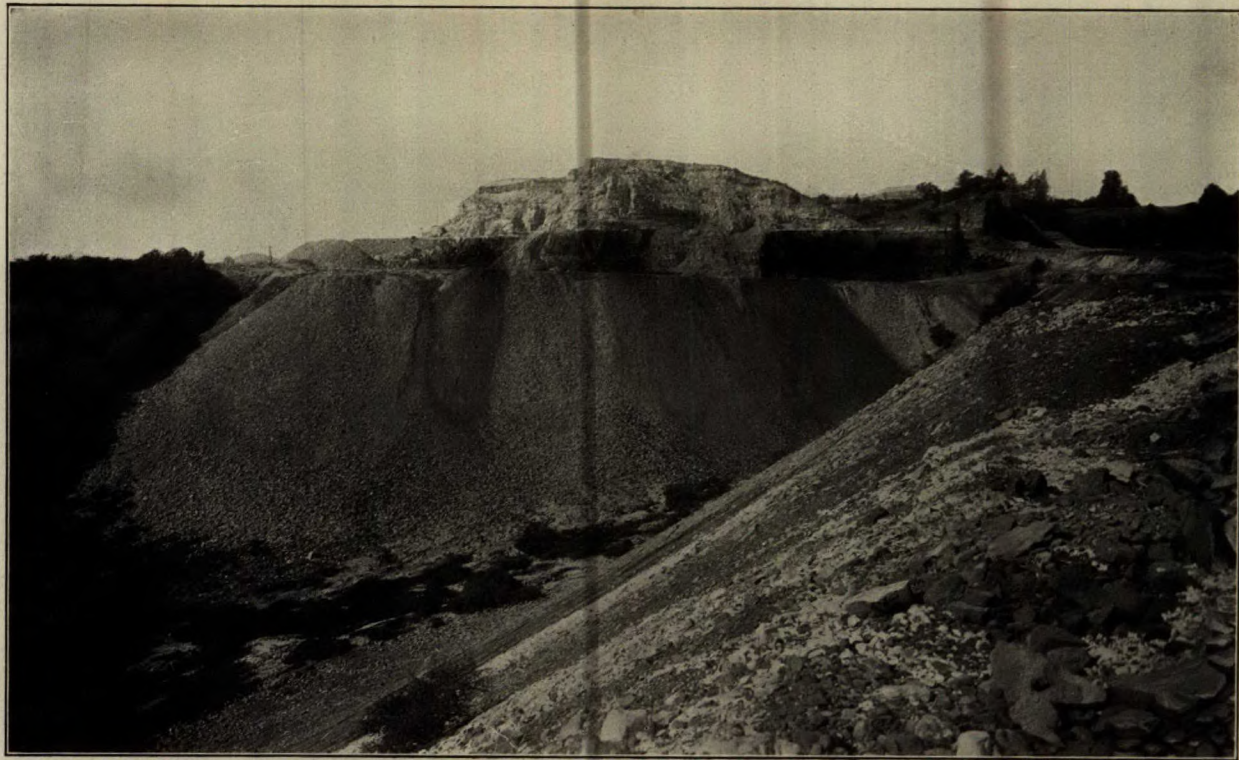
Bituminous sand quarry, near Godola, Cal. Thickness of 15% bituminous sand 60 feet; thickness of rock overburden 60-70 feet.
