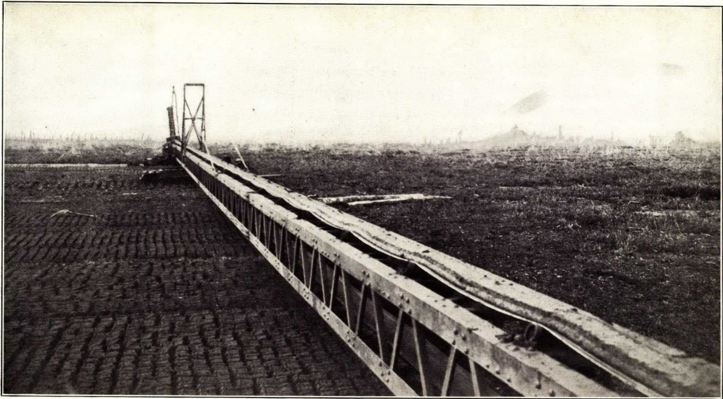
Belt conveyer with spreader in position near the end farthest removed from the line of excavation, and the entire plant at the end of the working face ready to be reversed
