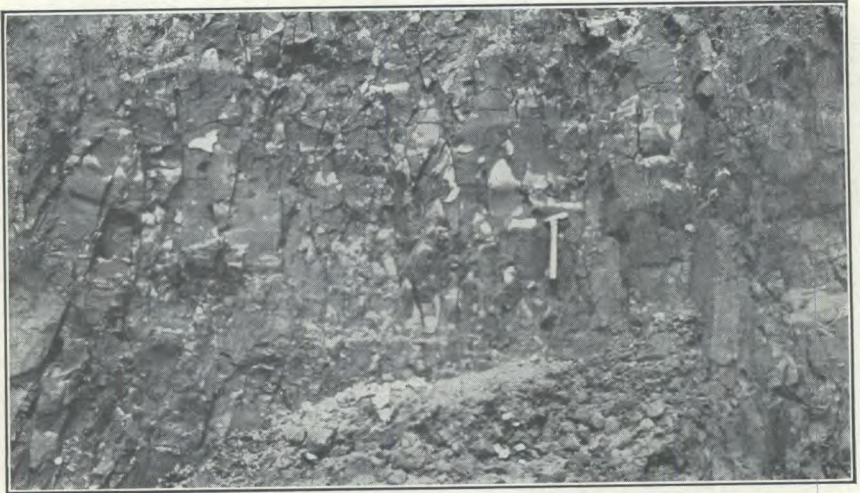
Typical exposure of freshly excavated upper marine clay in St. Lawrence valley.
