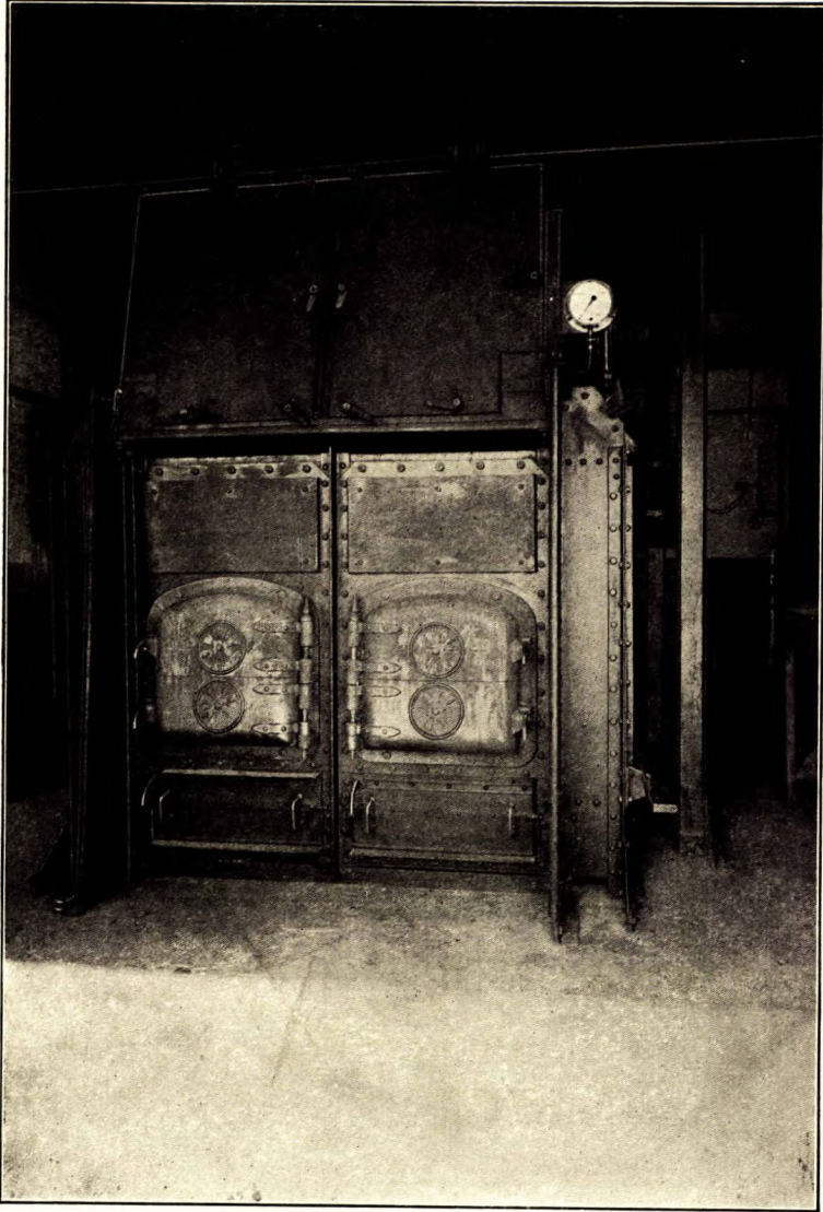
Fuel testing station: boiler room.
