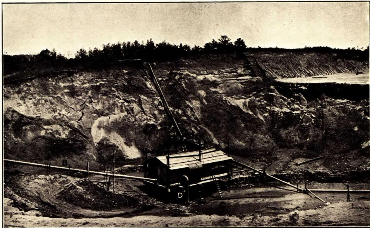
Hydraulic stripping at Rowe mine, Minnesota. (A) Water supply pipe to hydraulic gun. (B) Discharge pipe from centrifugal pump. (C) Sump. (D) Suction pipe connected with centrifugal pump.
