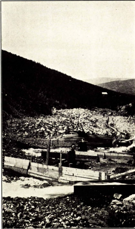
Maier's placer workings on Victoria gulch. Lone Star mill in the background.
