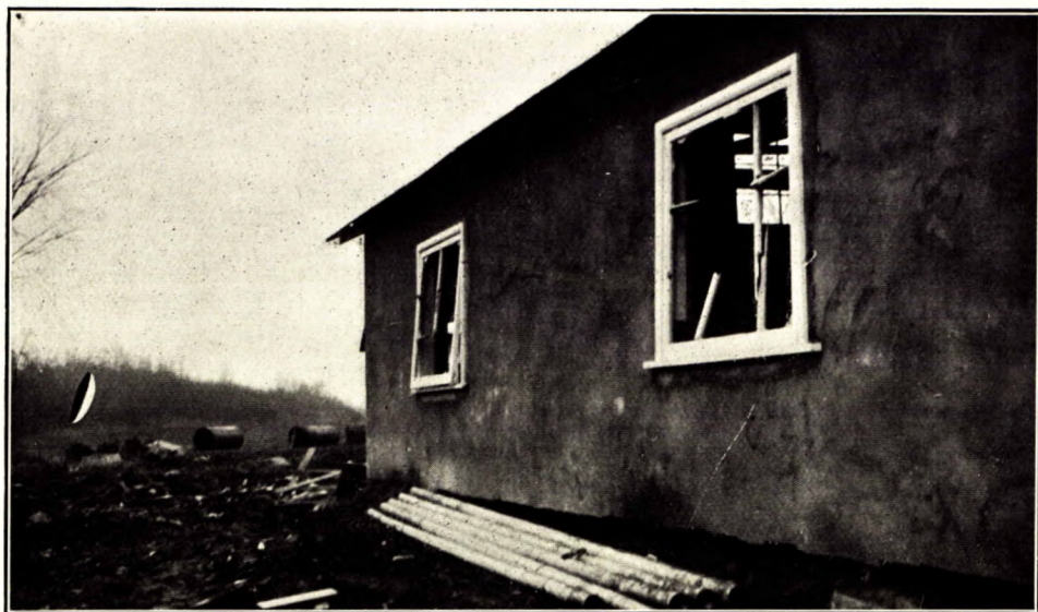
Explosion of one ton of 60 per cent dynamite. This house is one of the buildings at the acid plant, about 600 yards from mixing house. Building constructed of reinforced concrete. See effect of suction.
