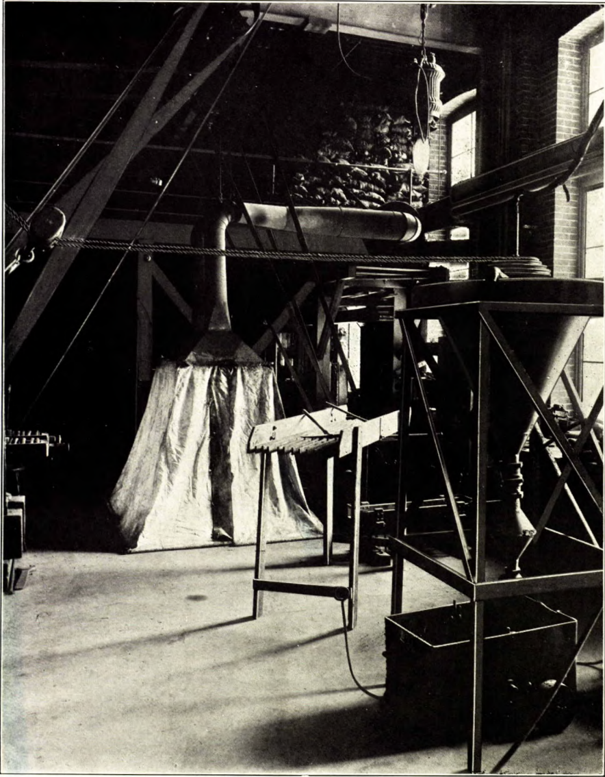
Crusher platform, bar screen, Robinson washer, and dust exhaust. Department of Mining and Ore Dressing, McGill University.
