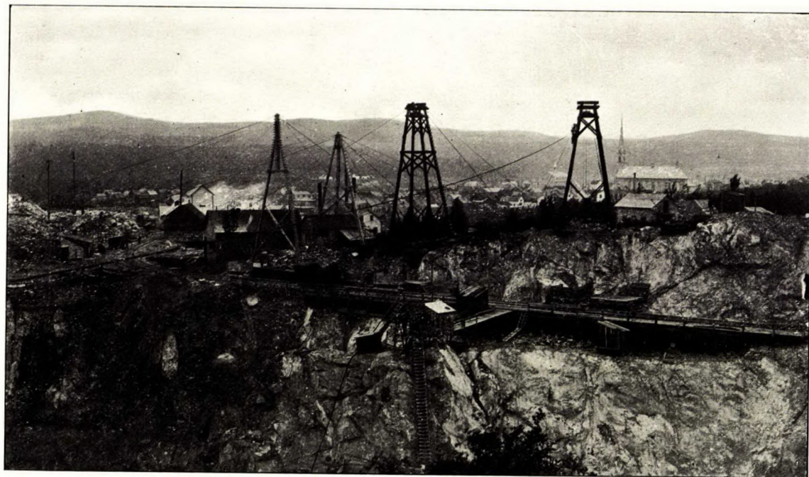
Arrangement of Cable Derricks and Tracks near Border of Pit. King Bros.' Mine, Thetford.
