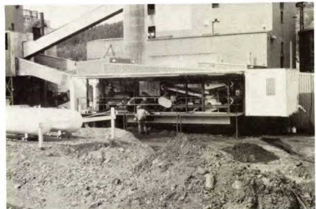
CANMET's mobile dewatering plant No. 2 at a coal washery
