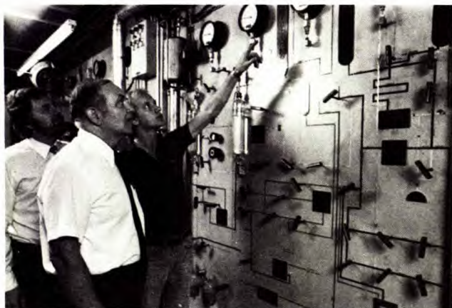
Researchers D. Patmore (L), and M. Pleet (R) discuss operation of CANMET's hydrocracking l-b/d pilot plant with plant operator A Kuiper
