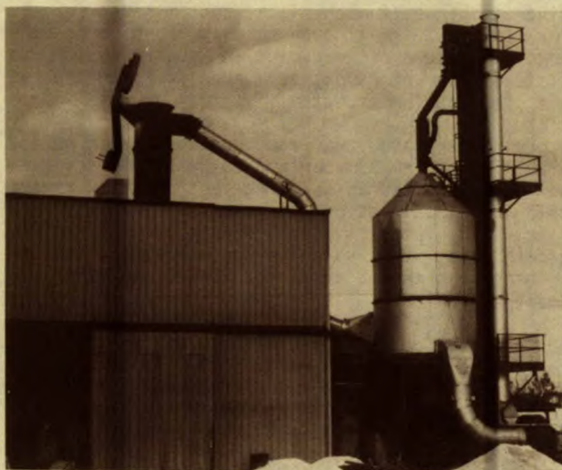
Fig. 30 - CANMET packed-bed filter installation on foundry cupola stack
